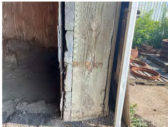
Photo 18 – Damaged Wood Siding
