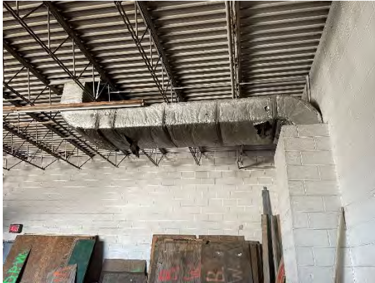
Photo 2 – Damaged Ductwork Insulation
