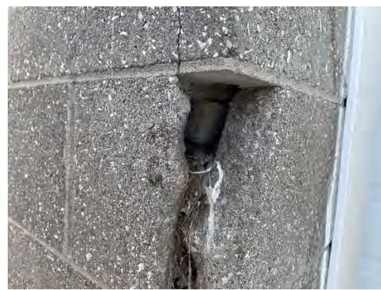
Photo 6 – Deteriorating Exterior CMU Wall
