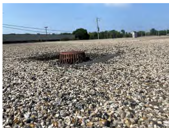
Photo 6 – Aging Ballasted Roof Membrane
