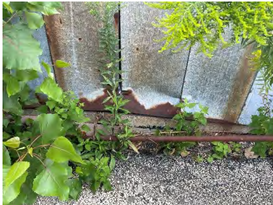
Photo 9 – Damaged Metal Siding
