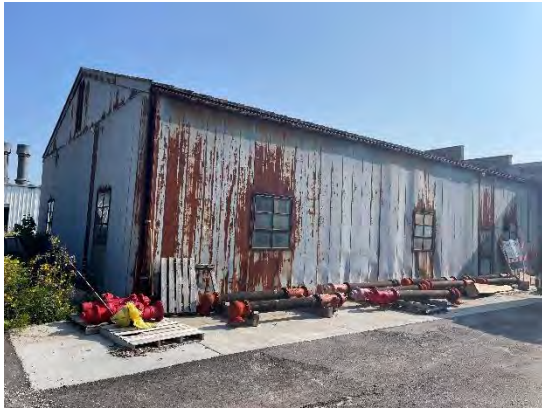
Photo 7 – Corroding Metal Siding
