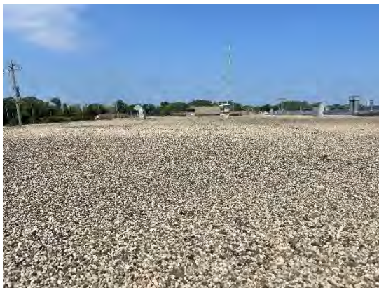
Photo 5 – Aging Ballasted Roof Membrane
