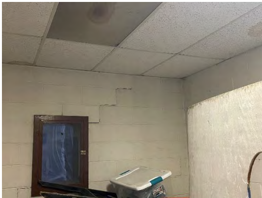
Photo 3 – Cracking Interior CMU Wall
