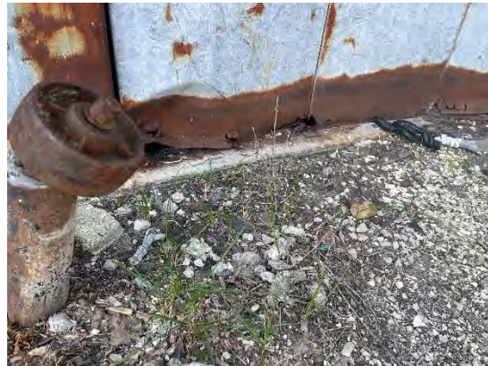
Photo 8 – Corroding Metal Siding
