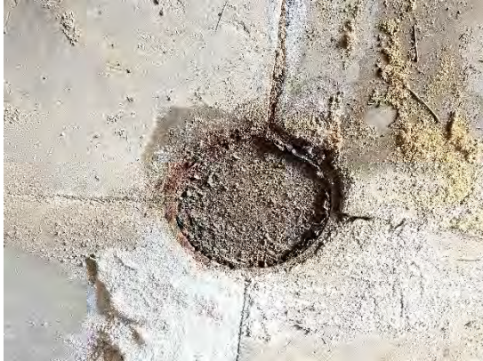
Photo 1 – Floor Drain Blockage
