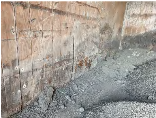
Photo 17 – Damaged Wood Siding
