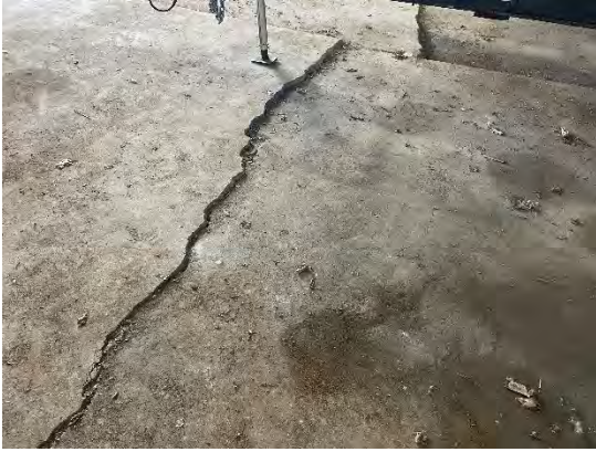
Photo 1 – Cracking Interior Concrete Slab
