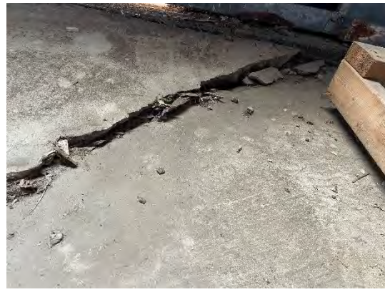
Photo 2 – Cracking Interior Concrete Slab
