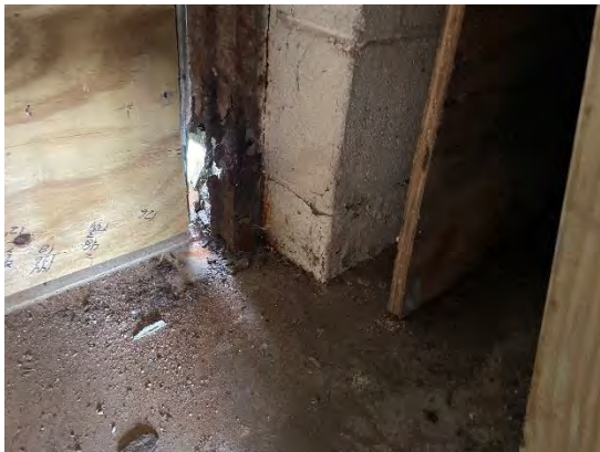
Photo 15 – Corroding Metal Door Frame
