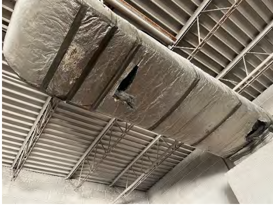
Photo 1 – Damaged Ductwork Insulation
