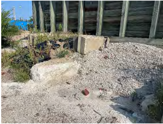
Photo 7 – Damaged Concrete Bin Blocks
