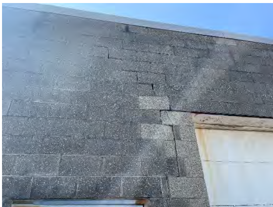
Photo 5 – Cracking Exterior CMU Wall
