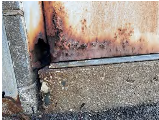
Photo 14 – Corroding Metal Door Frame
