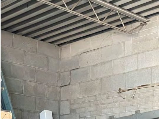
Photo 1 – Cracking Interior CMU Wall
