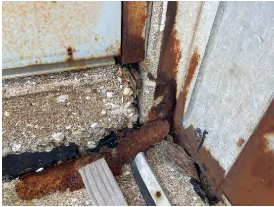
Photo 13 – Corroding Metal Door Frame
