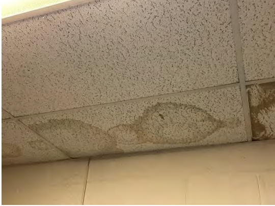
Photo 5 – Stained Ceiling Tiles
