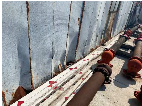
Photo 10 – Damaged Metal Siding
