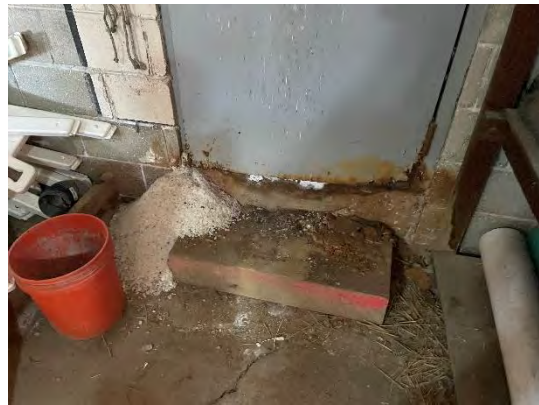
Photo 16 – Corroding Metal Door
