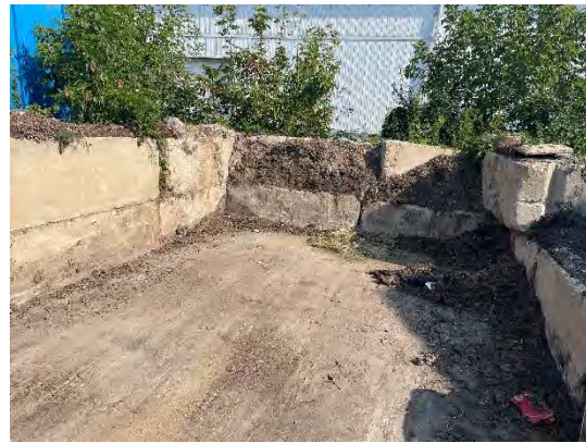
Photo 8 – Damaged Concrete Bin Blocks
