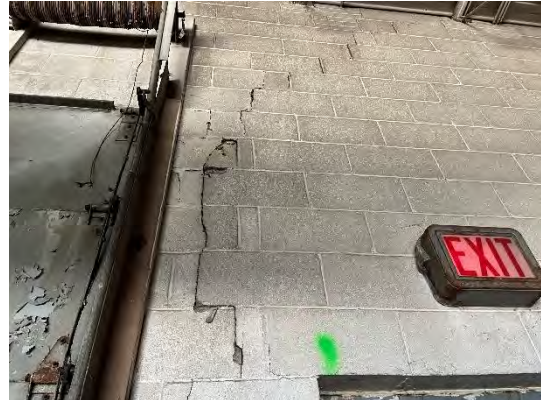
Photo 2 – Cracking Interior CMU Wall
