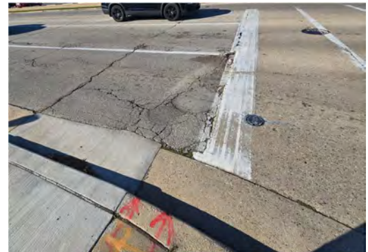
6. Deteriorated pavement at the intersection, illustrating the need for rehabilitation to improve drivability.
