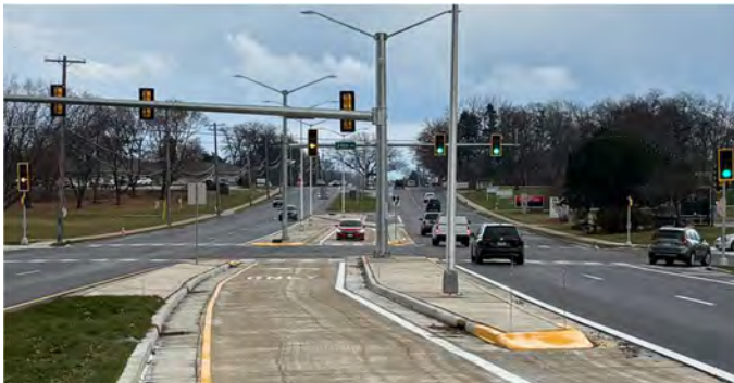
Following completion, there are now channelized left-turn lanes that eliminate the negative offset, monotube signals with reflective backplates and flashing yellow arrows, and enhanced pedestrian facilities.
