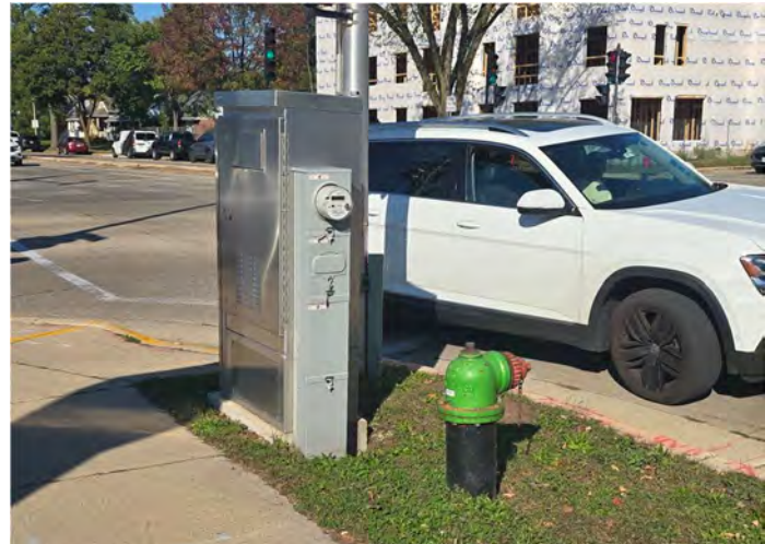
9. Traffic signal cabinet in vulnerable location.
