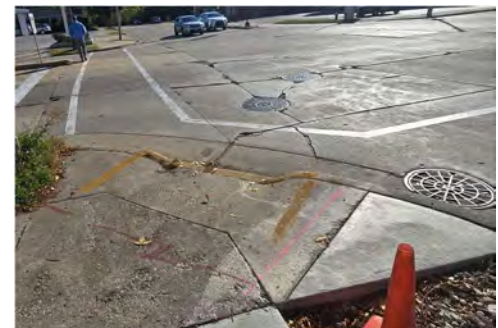
3. Substandard curb ramps in all four quadrants of the intersection.
