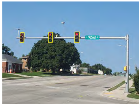
Monotube signals with lane-designated heads, reflective backplates, and flashing yellow arrows offer improved visibility.
